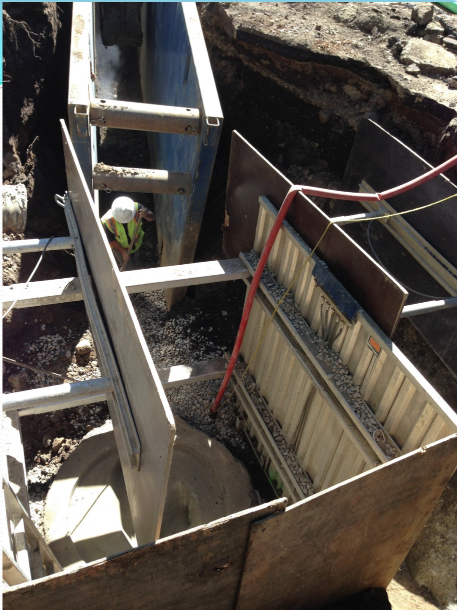
New sewer manhole base, ready for barrels and cone to be stacked; trench box; shoring
