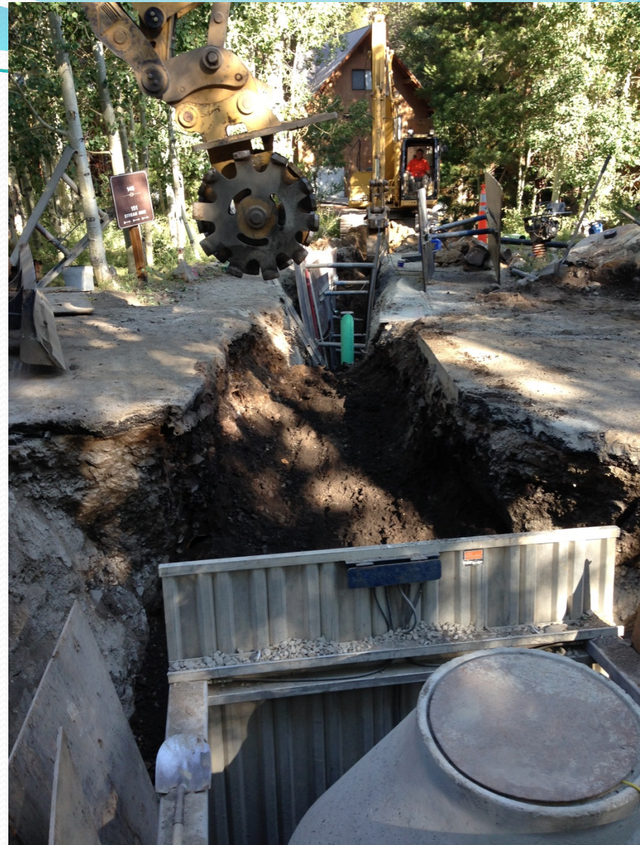
New sewer trench alignment with compacted backfill; new sewer line; shoring; new sewer manhole
