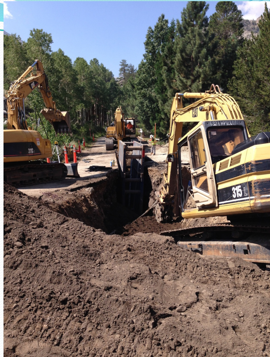
Multitask sewer installation: trenching and installing new sewer line followed by trench backfill and compaction
