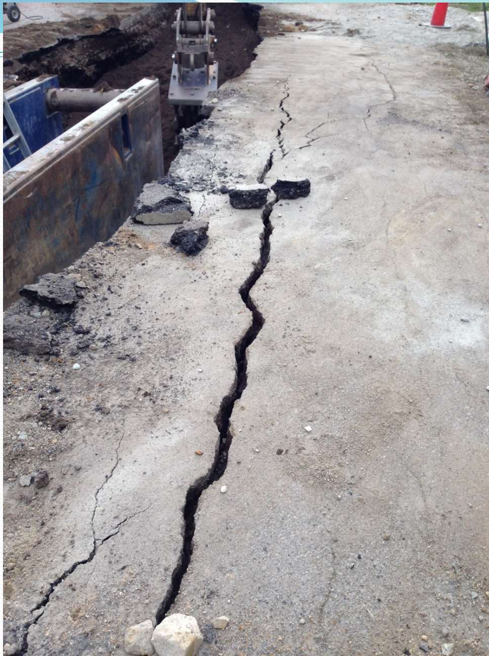
Existing pavement failure due to weak subsoil adjacent to sewer line trench
