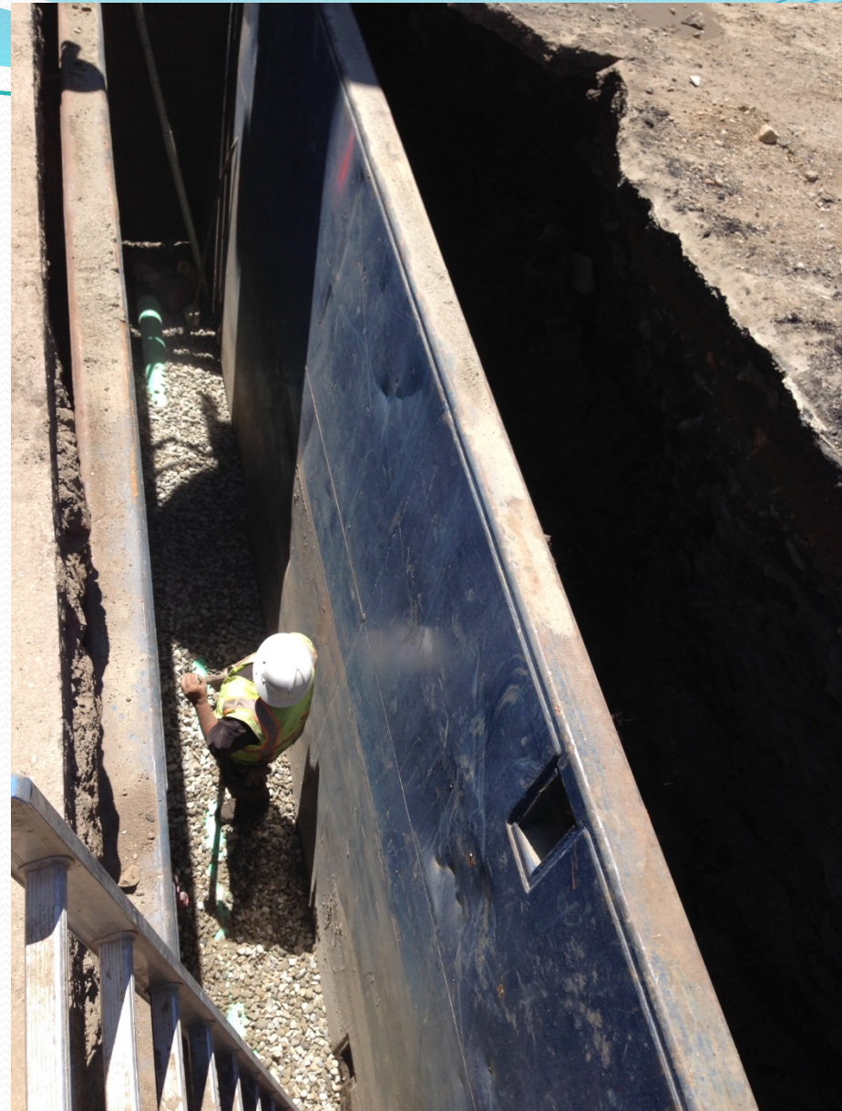
New sewer line in deep trench with rock shading and trench box shoring
