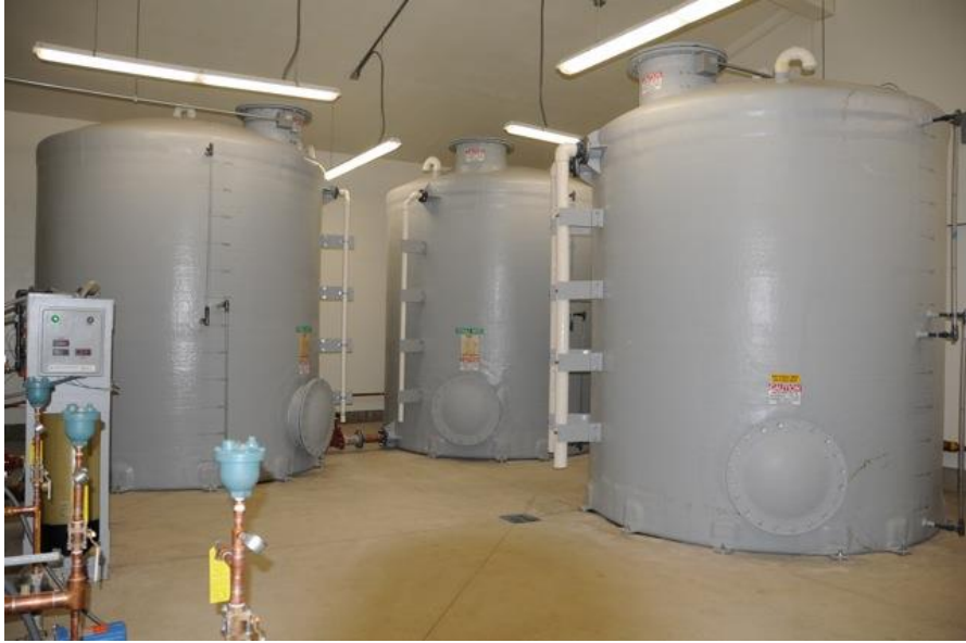
6,800-gallon water storage tanks
