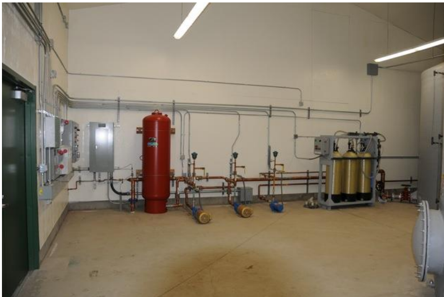
Domestic water supply pumps and Ion exchange treatment unit
