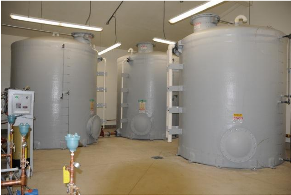
6800 gallon water storage tanks
